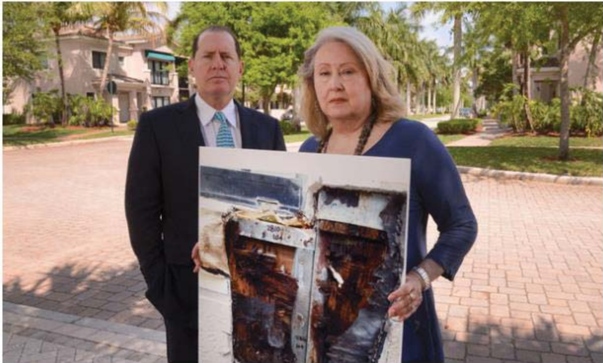
San Matero condo association's Jackie Durham holds an image of the the condition of the walls at a building there with attorney David Haber.
